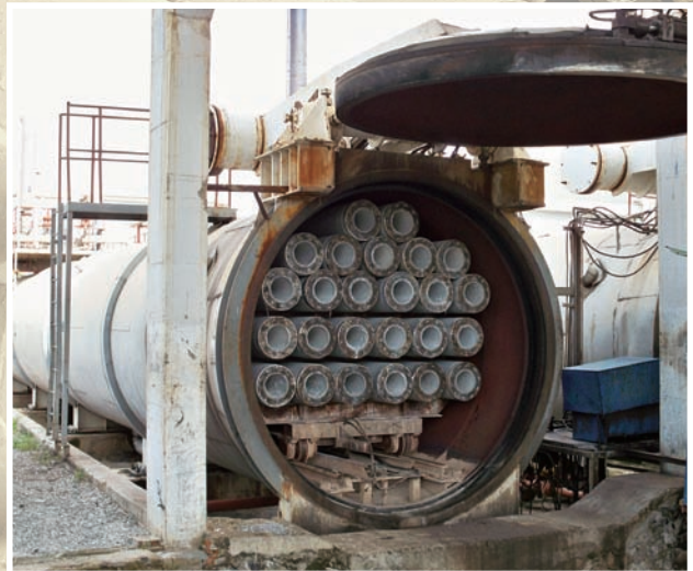
高溫高壓養生爐 Autoclave curing stove
